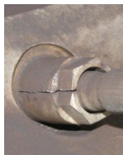
Sensor with cracked nut
